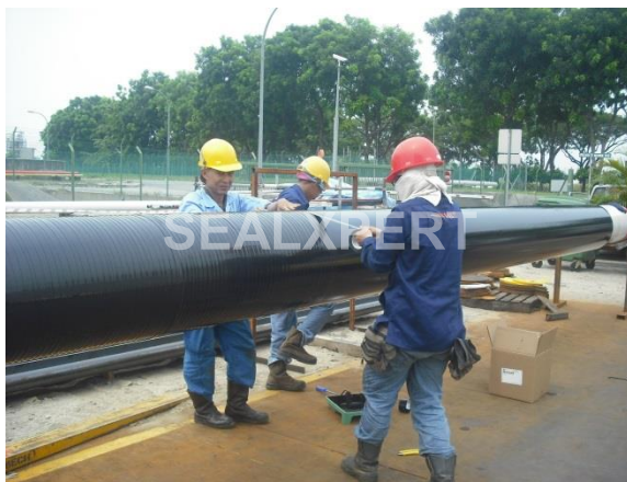
Fig 2: Wrapping of the first layer of SealXpert Poly Inner Wrap around the pipe
